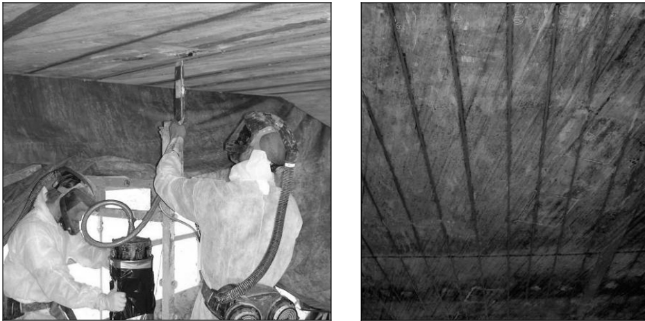
Figure 7.12 Left: Application of epoxy in an NSMR groove; Right: Final appearance of the bridge's underside after insertion of bars and removal of tape
