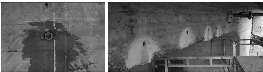
Figure 7.14 Left: Drill head exiting the bridge; Right: Entrance holes when the drilling process is finished
