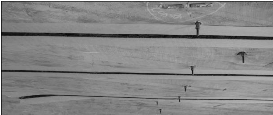
Figure 7.11 Picture from underneath the Frövi Bridge with the NSMR grooves primed, taped and ready for application of epoxy and bars
