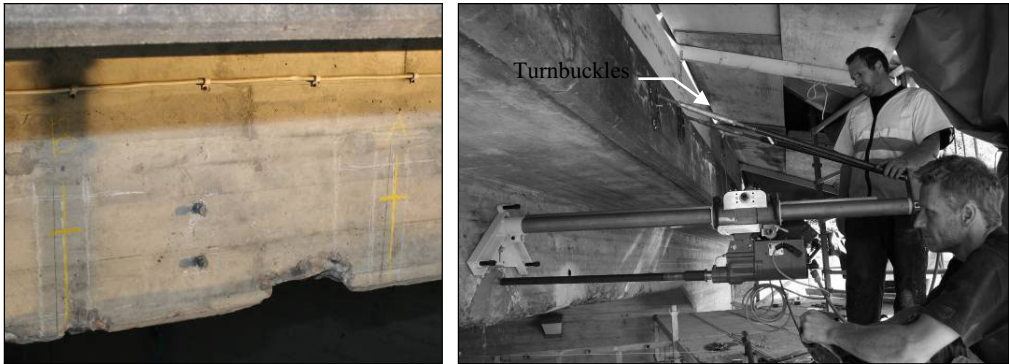
Figure 7.13 Left: Hole positions marked in yellow and near surface steel reinforcement in white chalk; Right: Drilling equipment
